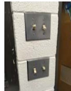
Typical Light Controls
