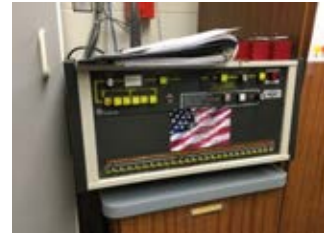
Existing Intercom Head-End
