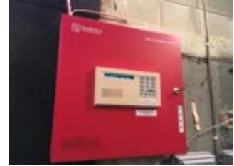
Boiler Monitoring System
