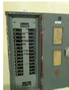
Old Branch Panelboard
