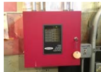
Fire Alarm Control Panel
