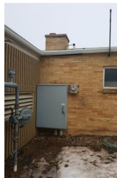
C/T Cabinet & Meter
