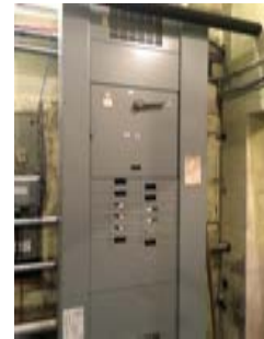
Main Electric Service
